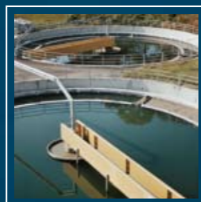
Waste Water Treatment Plant
